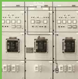
LV Power distribution
