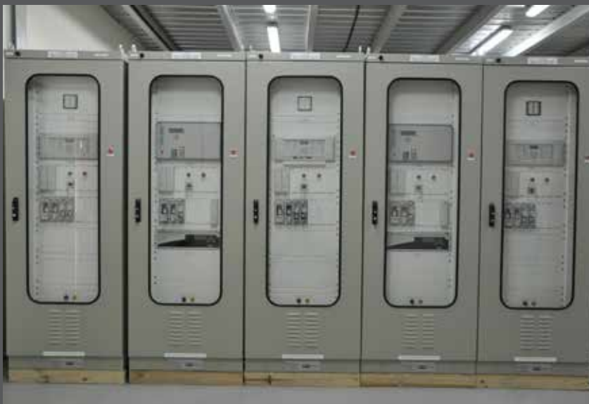
400kV Protection Panels at Ajman Grid Station for ADWEA, UAE.
