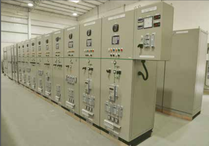
33kV Combined Control & Relay Panels at Aziaba North-3 Primary Station for MEDC, Oman
