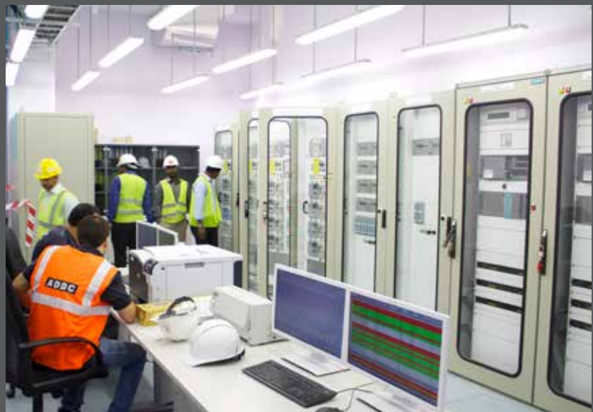
12MVAR, 22kV Capacitor Bank Control & Protection Panel SAT testing for ADWEA, UAE
