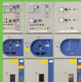
MV Power distribution
